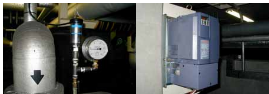
Inverter-control with pressure sensor
